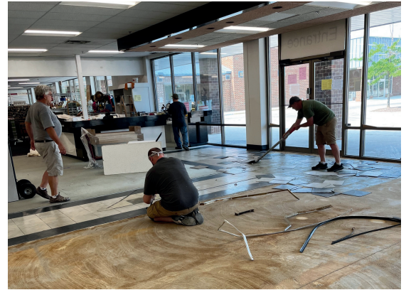
Many volunteers invested countless hours to accomplish the renovation project on time and within budget.
